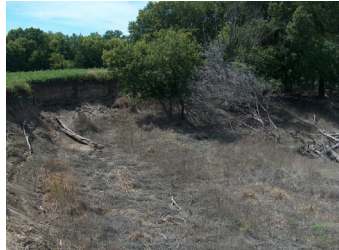
Grand Marais Outlet Restoration Project of the Red Lake WD, looking west at erosion area upstream of the Red River of the North.
